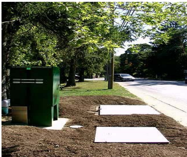
The yellow feature in the first photo is the Rentricity innovation that captures excess pressure in water systems and converts it into power. The middle photo shows the electrical tie-in. The final photo shows the finished application of the new technology.
